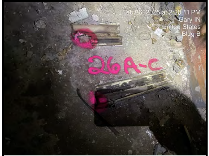
Sample # B-Base-26 Pipe Insulation - 0"-6" Duplex Insulation
