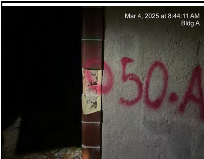
Sample # A-50-Bas Ceramic Tile with Grout and Mortar - Walls, 2"x4" Dark Red and Beige
