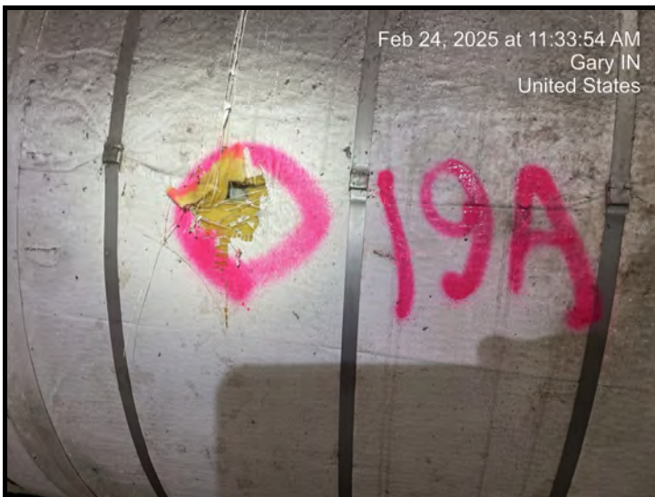
Sample # C-B-19-A-C Tank Insulation - Fiberglass with Foil- Tank 1
