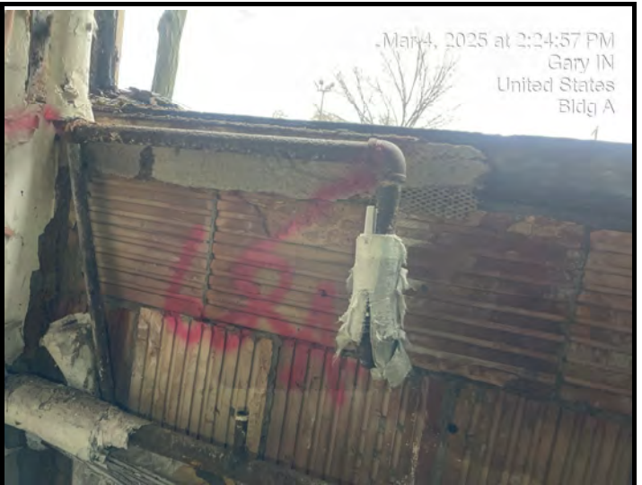
Sample # A-68-Bas Pipe Fitting - 0" -6" O.D. Mudded pipe fitting Insulation on Air Cell SRPI
