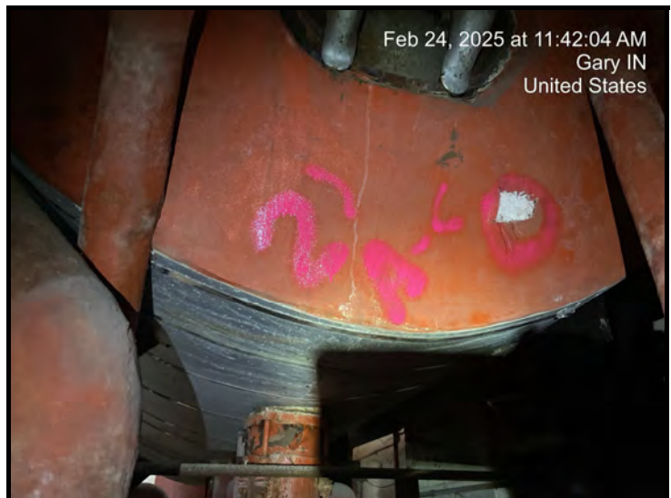
Sample # C-B-21-A-C Tank Insulation - Fiberglass with Foil Paper- Tank 3
