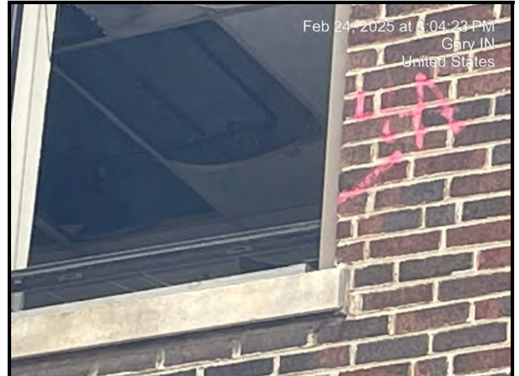
Sample # C-Ext-4-A-C Exterior Caulk - Around Aluminum Window Frames- 2nd floor
