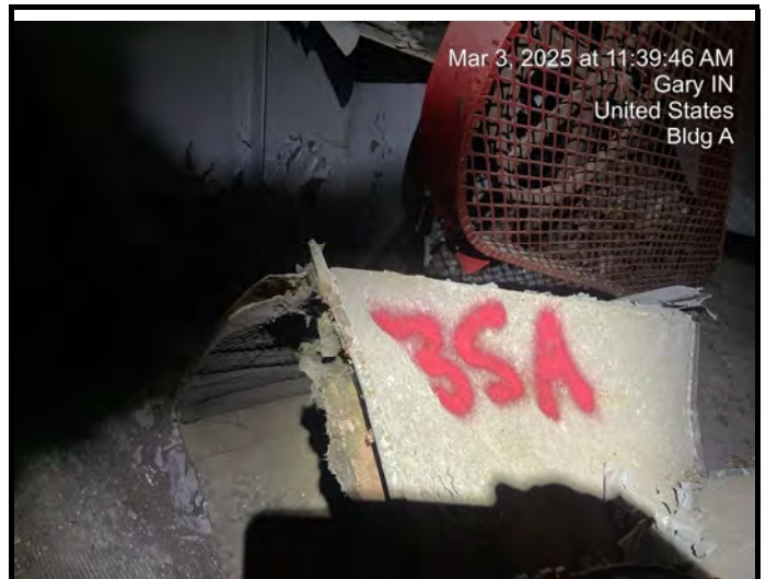
Sample # A-35-Bas Duct Insulation - Interior of Ductwork
