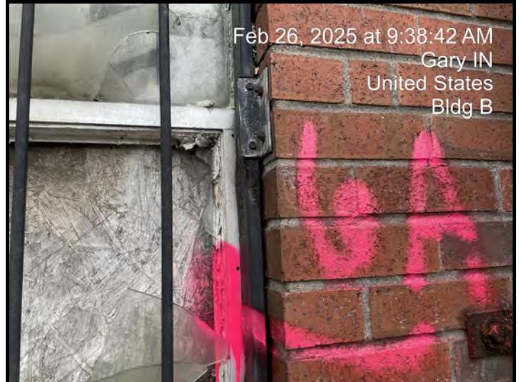
Sample # B-Ext-6 Window Glaze - Metal Framed Windows, Basement, 1st, 2nd
