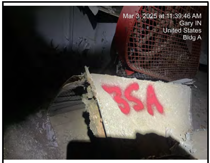
Sample # A-35-Bas Duct Insulation - Interior of Ductwork
