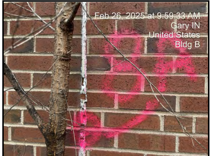
Sample # B-Ext-8 Exterior Caulk - on Brick Siding, former awning
